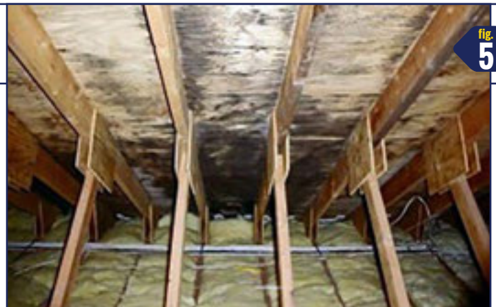
Moisture problems can often lead to mold issues as shown in this attic.
