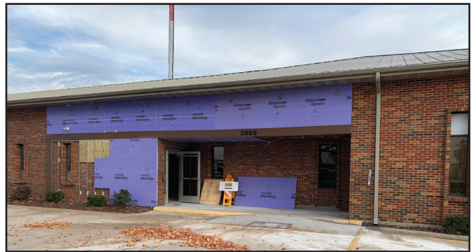
By the time you receive this month's newsletter, the front of the building will most likely be complete! Here is a photo during the reconstruction, which included masonry repairs and a facelift to our existing entrance.
